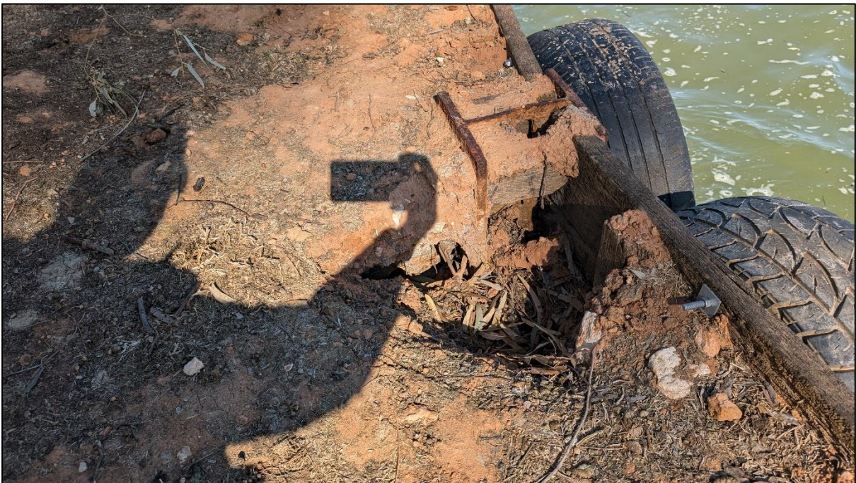
Figure 4: View of the existing retaining wall damage
