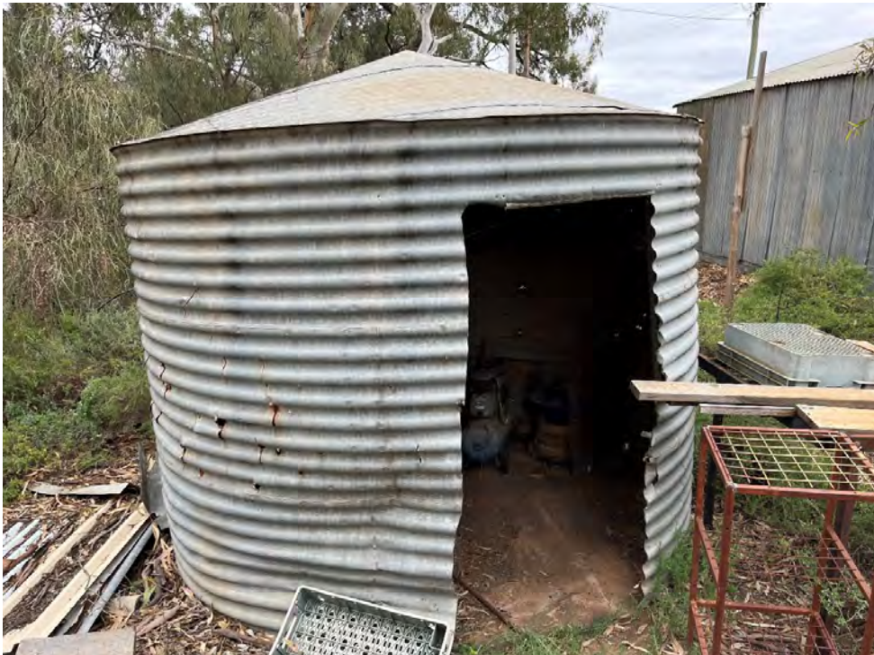
Photo 32. Lot 3 DP236223 Old rainwater tank purposed for storage of generators and pesticides
