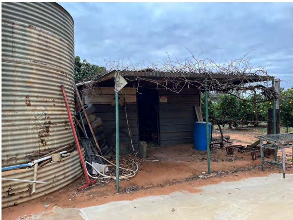
Photo 2. Lot 1 DP125848 Former chemical storage shed and water tank (both now disused)
