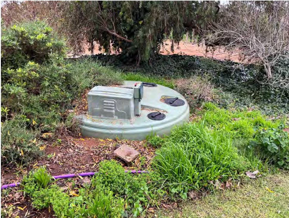
Photo 11. Lot 1 DP1269246 Septic Tank
