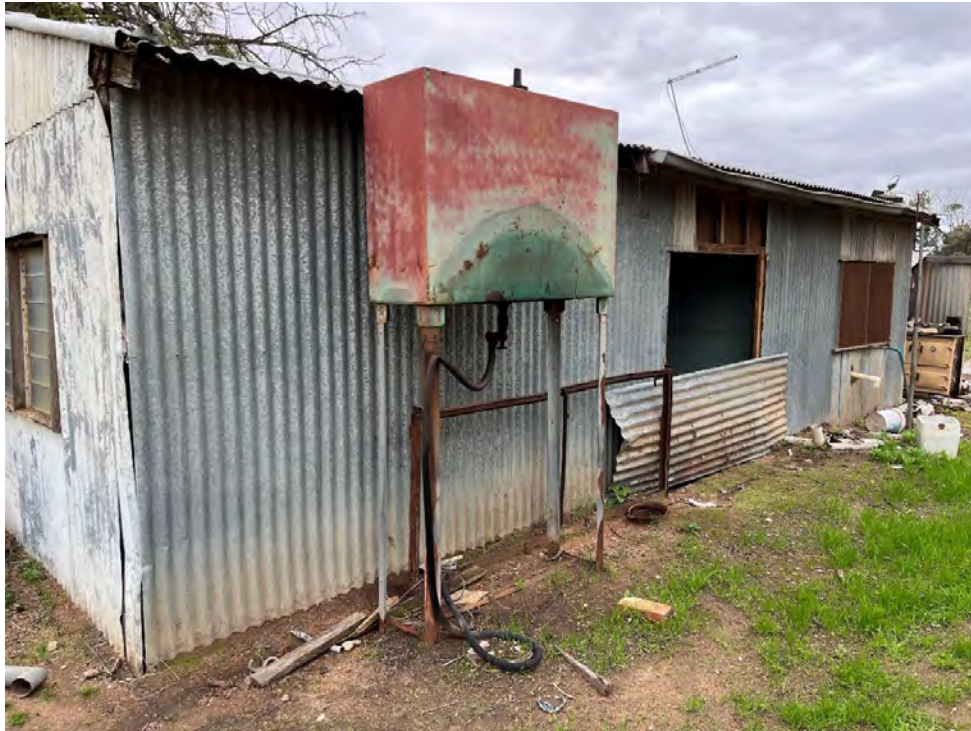
Photo 39. Lot 5 DP236223 Former heating oil tank converted to diesel (now disused)
