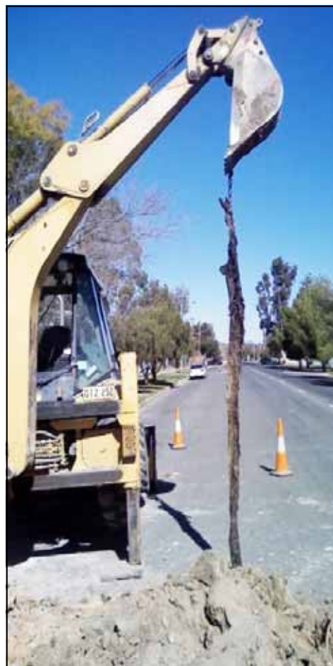
These 3.5 metre long roots were removed from one of the old earthenware sewer mains on Wednesday 27th August.
