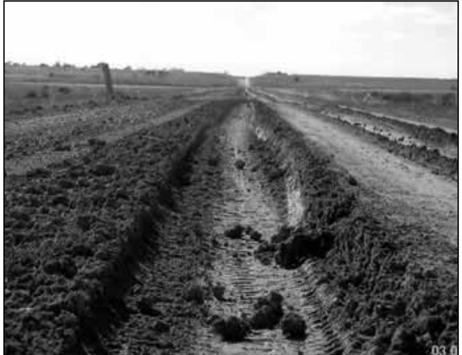
Typical damage, this time to the Pooncarie to Ivanhoe Road, caused by a heavy vehicle travelling the road during, or too soon after, a rain event. This road was graded on a Thursday and destroyed on Friday!
